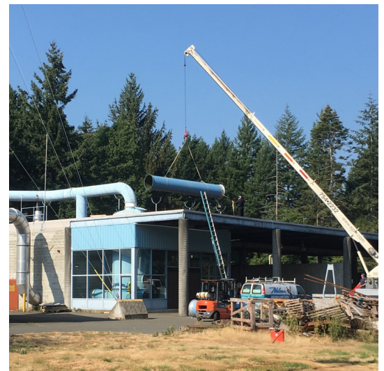
The existing air scrubber – which cleans the air of odour – undergoes a retrofit.
