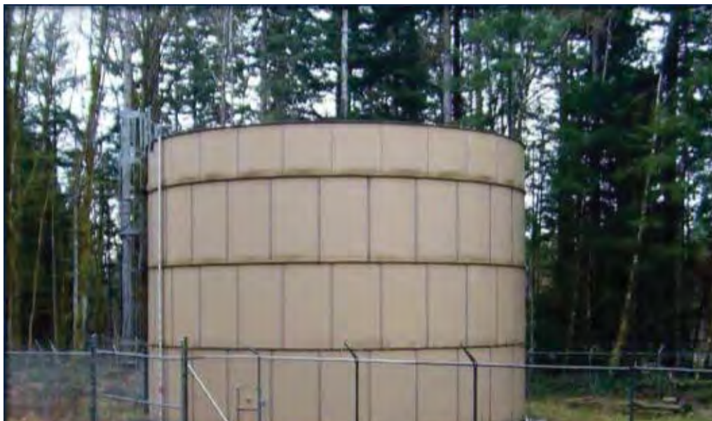
Mitchell Road Storage Reservoir – if conversion is approved, the reservoir will be decommissioned. Koers Engineering recommends that a detailed review of the condition of the existing tank should be completed to determine if the tank is in suitable condition to be sold as a water storage facility or if the tank should be sold for scrap.
