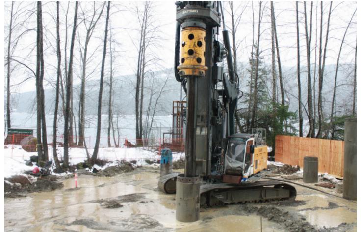
Through rain and snow the project team is moving ahead with drilling piles at the Raw Water Pump Station.
