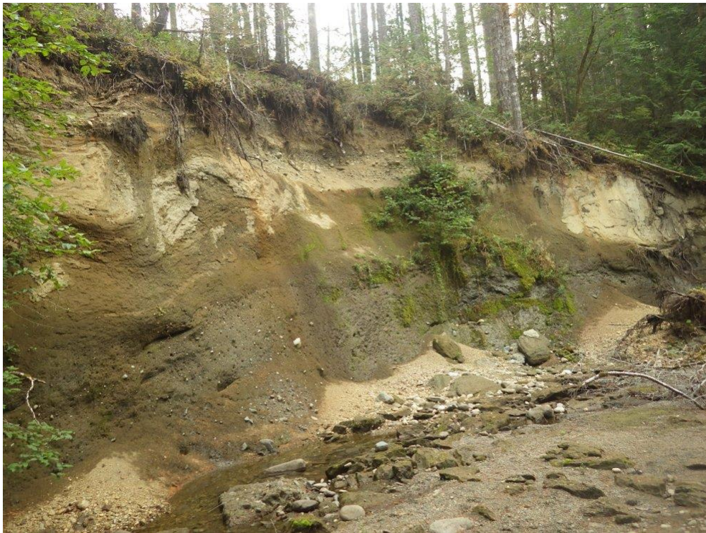
Figure 15. Eroding bank visible from Comox Lake Road, August 22, 2018.
