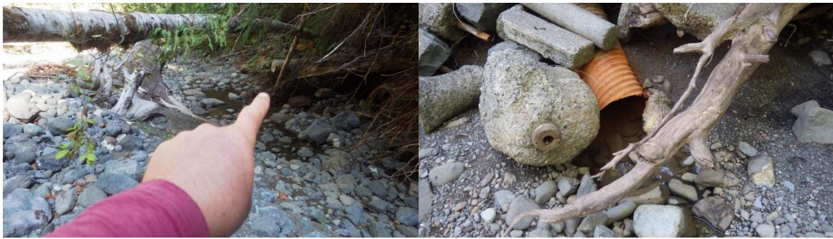
Figure 49. Water main drain, August 24, 2018.
