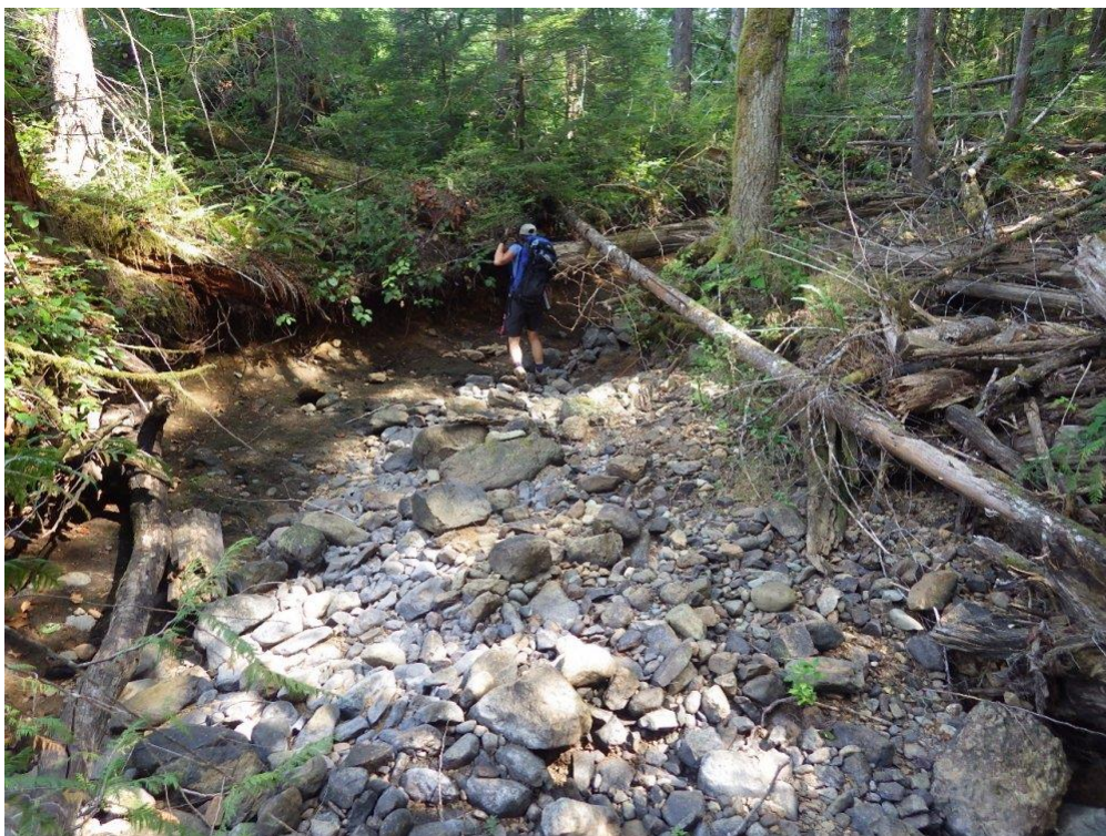
Figure 57. Severe erosion over 50 m x 2.5 m area, August 24, 2018.
