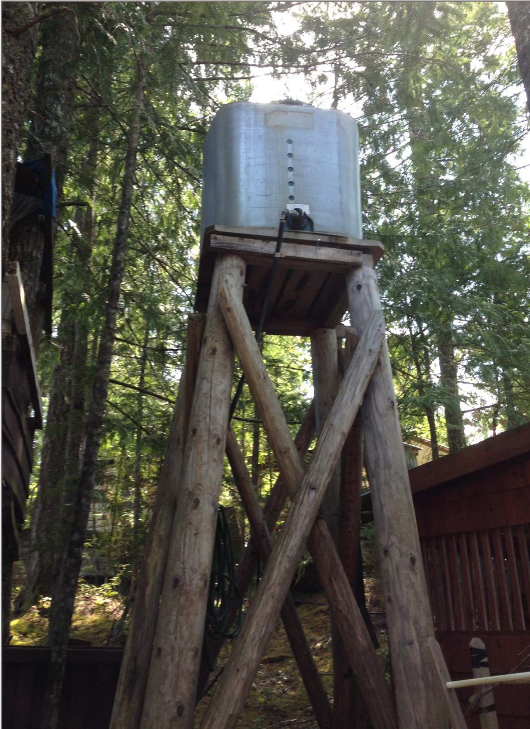
Photo 13: Potable water tank for a cabin on the north portion of the Property.
