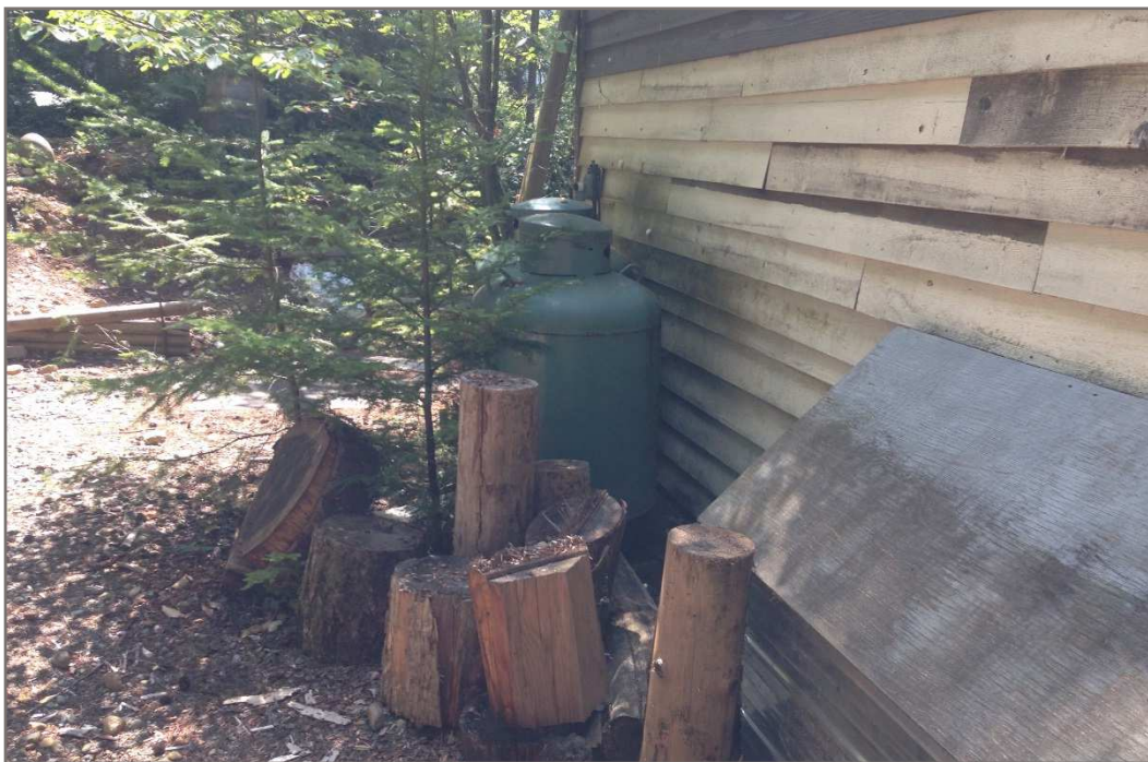
Photo 12: Twin propane tanks at a cabin on the north portion of the Property.
