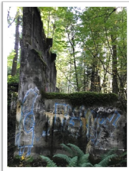
Figure 4 Concrete ruin of No.4 Mine Fan House showing exterior wall
