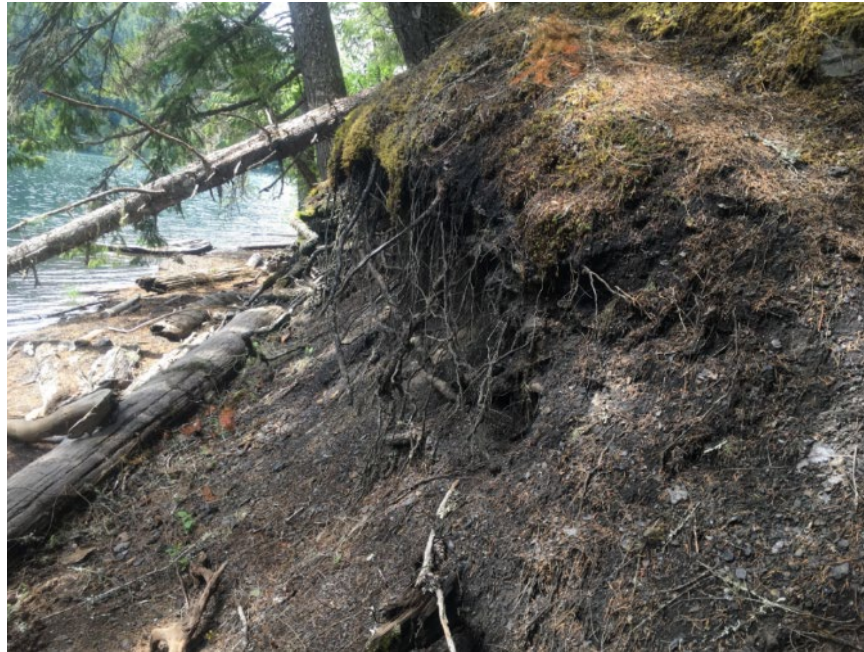
Figure 11. HBS11: Extensive erosion of coal slag along Comox Lake shoreline near Perseverance Creek, May 19, 2020.
