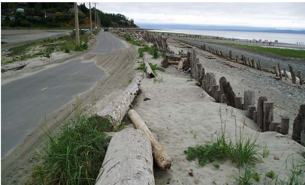
Photo 6: Sand Deposition on Road
