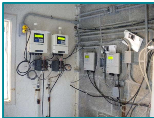
Figure 2: Chlorine Injection at the Royston Chlorination Station.
