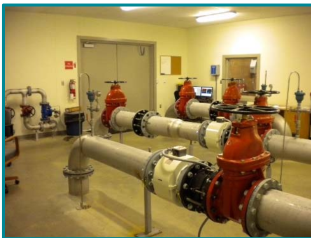
Figure 1: Inside the BCOB Water Treatment Facility.
