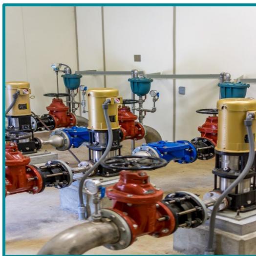
Figure No.1: Pump Station
