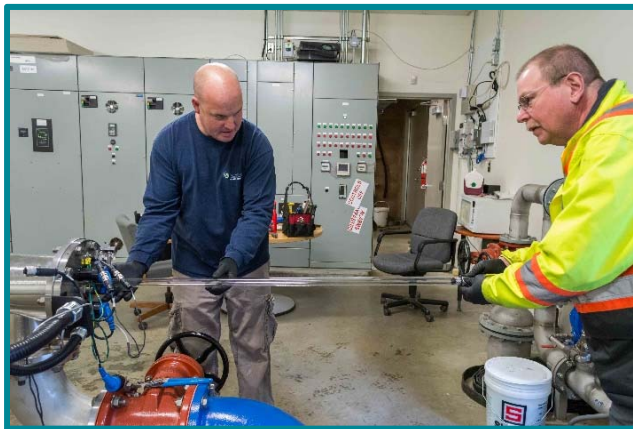
Figure No.1: Cleaning the UV bulb sleeves inside the BCOB Water Treatment Facility.
