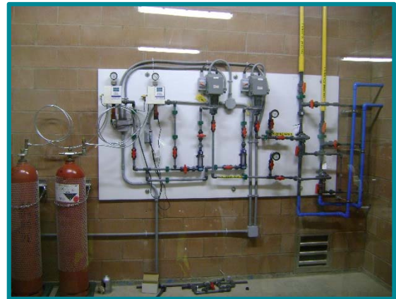
Figure No.2: Chlorine Injection within BCOB Treatment Facility
